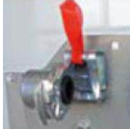
In-correct Application / Hatalı Uygulama
